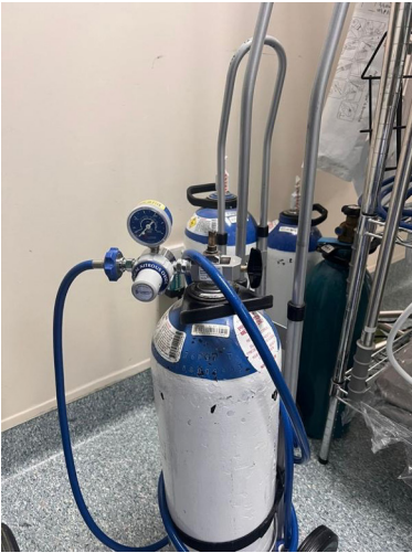
Figure 3. Portable N 2 O trolley systems
